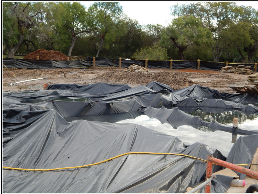
Figure 4-23. Water collected in the parking lot after heavy rains.
