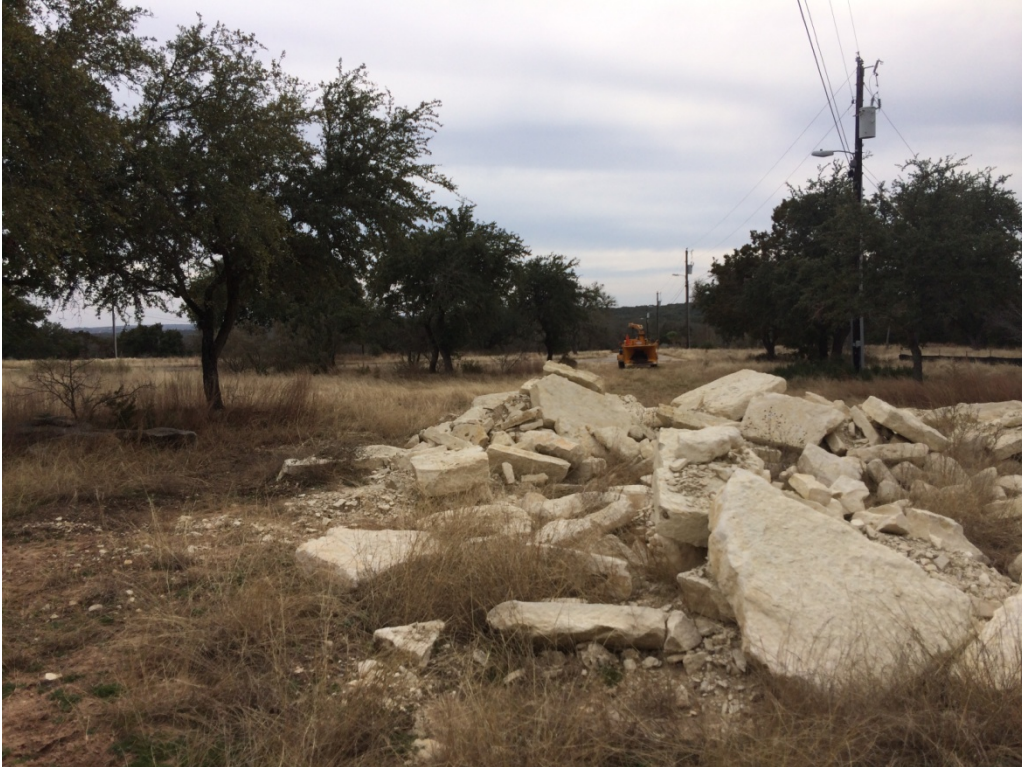
Figure 6: Demolished paved roadways and mobile home pads with construction equipment in background, facing south.
