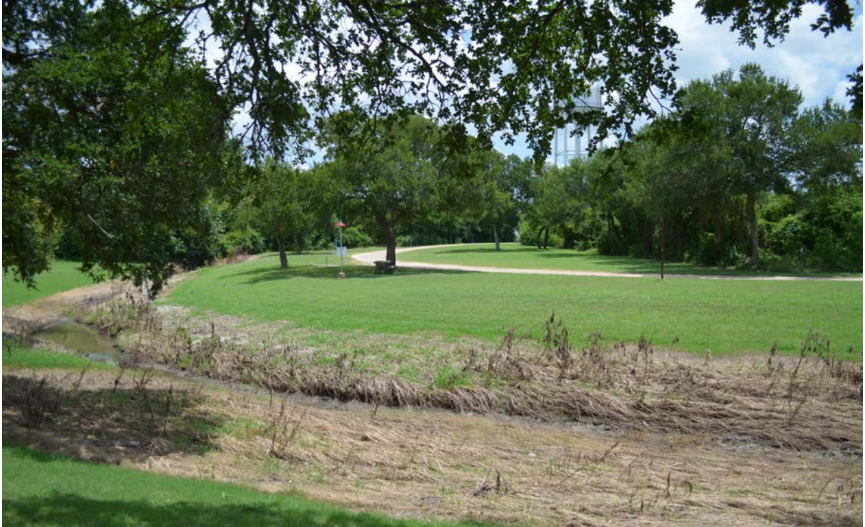
Figure 3. Northern view of Salt Creek that recently flooded in the park. Note previous channelization.
