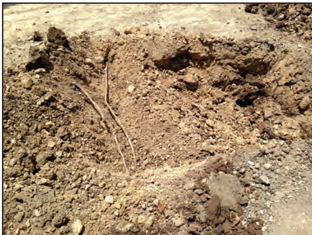
Figure 10.16. Example of braided grounding wires, adjacent to Pier 4, facing south.
