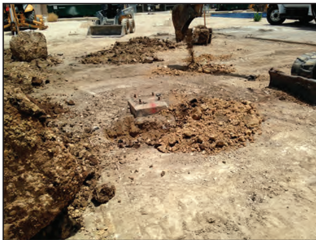
Figure 10.12. Example of existing pier foundation at surface to be removed; Pier 4, facing east.
