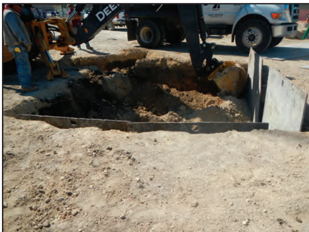
Figure 10.25. Facing southwest, installation of northeast and northwest shoring plates within manhole excavations, 13.9 feet wide.
