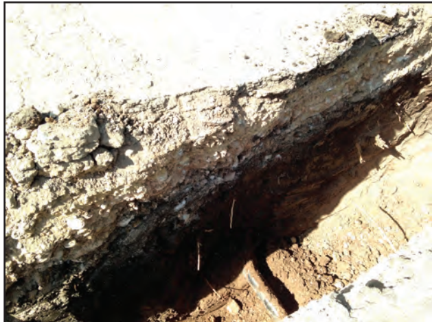
Figure 7.14. Existing CPS Energy gas line at north end of project area, facing south-southeast.
