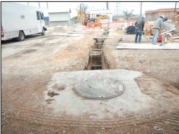
Figure 10.31. East end of duct bank trench excavations and existing manhole, facing west.
