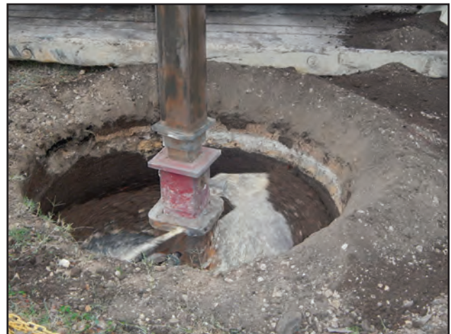
Figure 8.11. Upper horizon of Tower Location 10 disturbed from previous construction activities, facing east.
