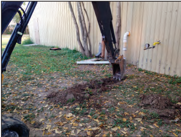
Figure 7.8. Trenching excavations on the south end of the project area, facing southeast.
