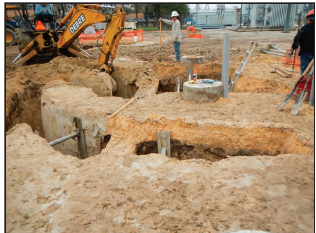
Figure 10.33. Two 8-foot extension trenches on the southern side of the west end of the duct bank trench, facing east.
