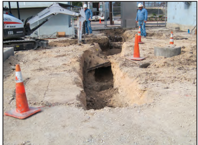
Figure 10.38. Overview of new conduit trench, located between Oil House and Control House, facing west.
