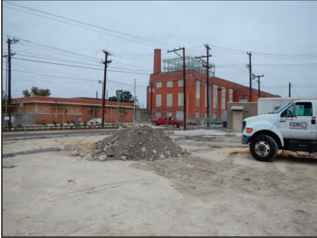
Figure 10.3. Mission Road Power Plant located to the northwest of the Ball Park Project, facing northwest.
