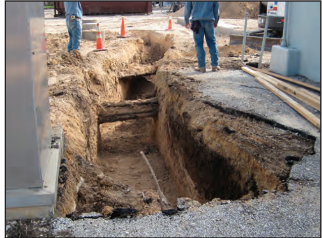
Figure 10.37. Facing east, overview of new conduit trench, located between Oil House and Control House, 5 feet deep.
