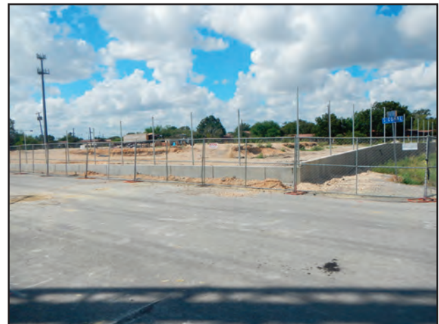
Figure 11.10. Overview of CPS Energy Comal Street Substation pad site, facing southwest.
