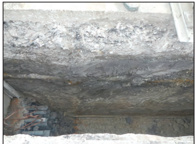
Figure 11.39. Existing cast-iron water main in profile of El Paso Street ROW, facing south.
