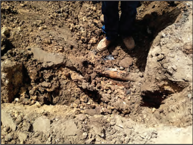
Figure 10.15. Example of PVC conduits, beneath Pier 2, facing south.
