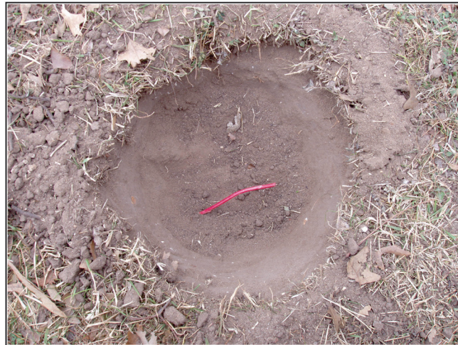
Figure 4-4. Shovel Test 3 where utility line was encountered.
