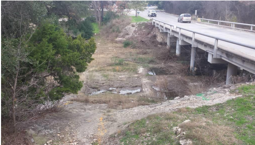
Photo #13: View north across Helotes Creek at point of proposed pedestrian bridge. Note the orange (center) and green (right) spray paint in the foreground marking buried fiber-optic and sewer lines, respectively.
