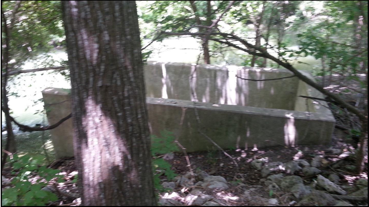
Figure 1-4. Existing outfall structure on eastern edge of Geronimo Creek that will be abandoned in place (photograph by Todd Schnakenberg).
