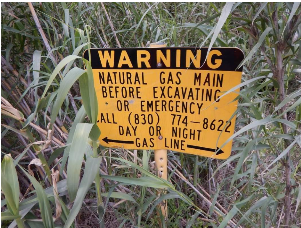
Figure 16. Buried gas line along the north side of Frontera Road in the southern half of the APE, facing north.
