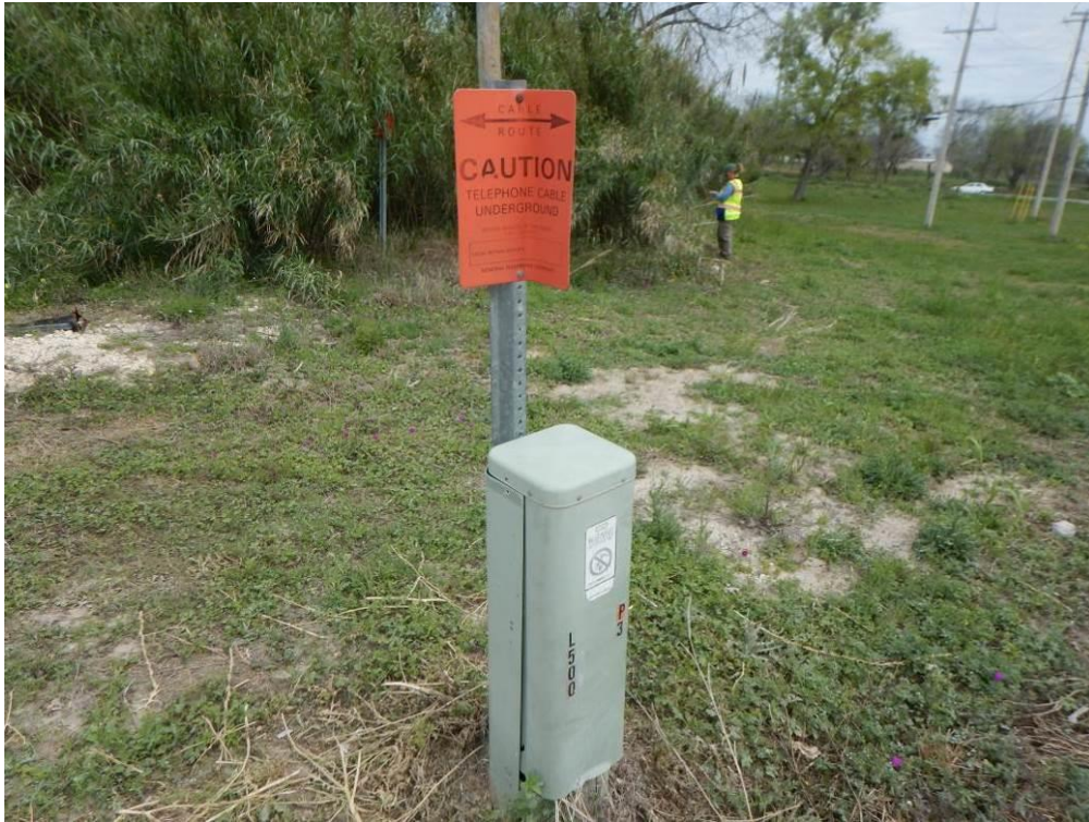
Figure 15. Phone line buried along the north side of Frontera Road in the southern half of the APE, facing east.
