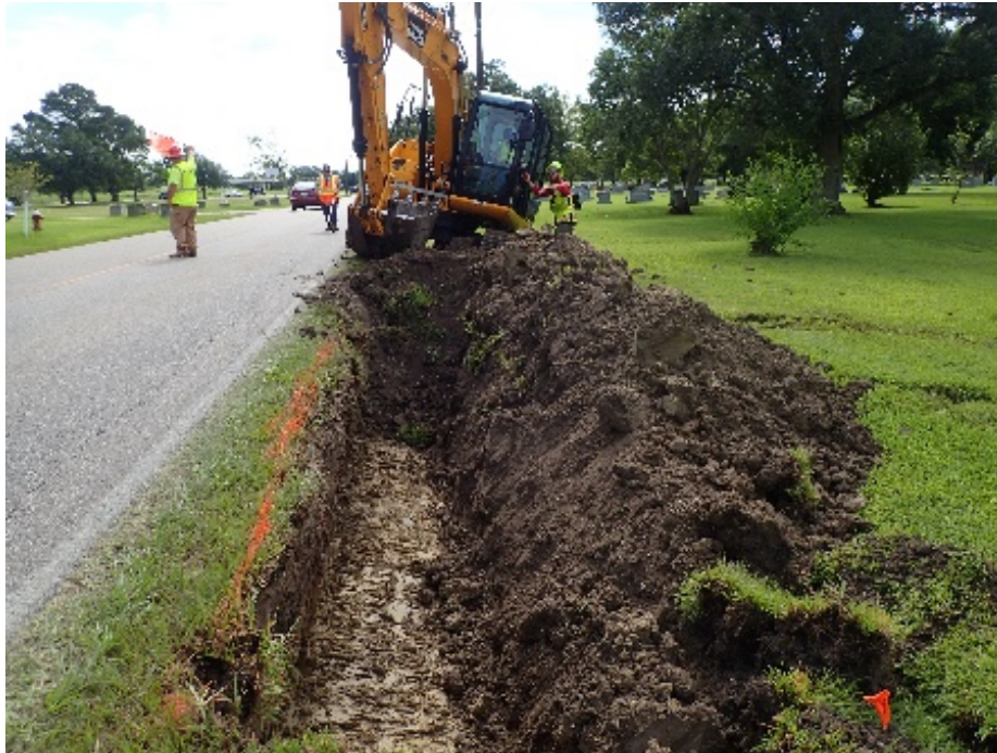
Figure 21. View of trenching south of FM 517, facing east. Note trench proximity to cemetery, flag indicating fiber optic line.
