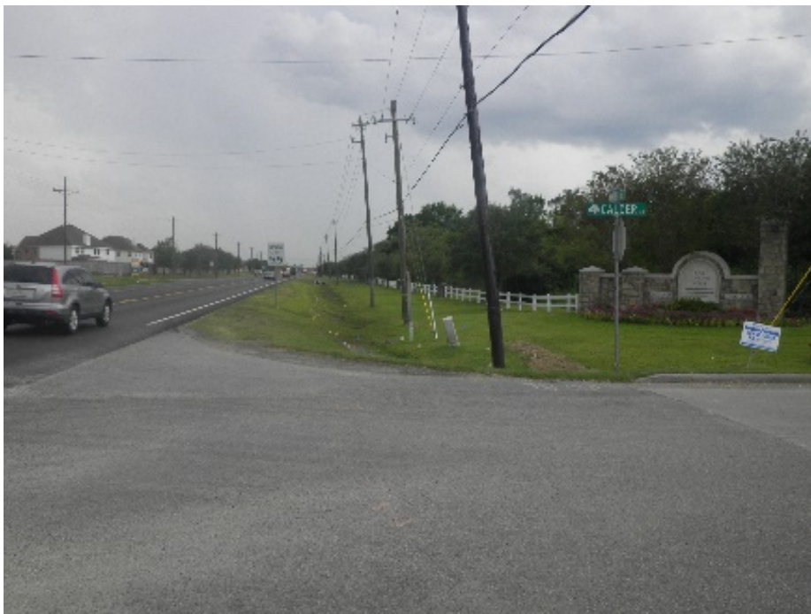
Figure 18. View of underground and above ground utility development, facing west. Note numerous pinflags marking subterranean utility installations.
