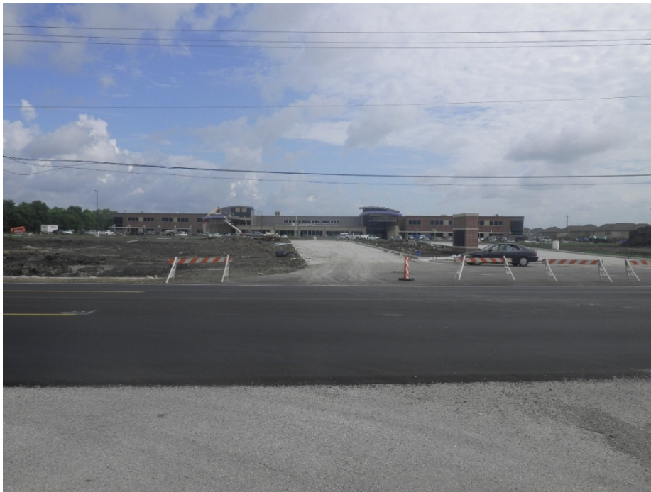
Figure 5. View of high school, under construction, facing north. Note highly-disturbed areas of remaining soils.
