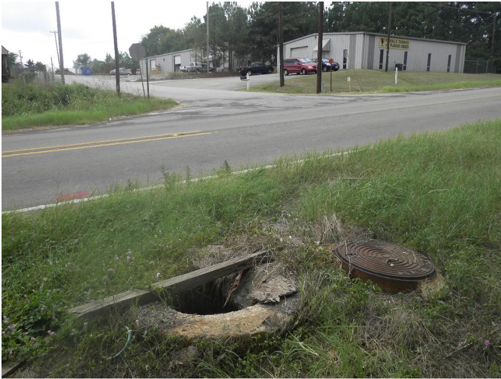
Figure 5. Evidence of subsurface utilities near unnamed drainage in APE with typical commercial enterprises in the background; view is to the north.
