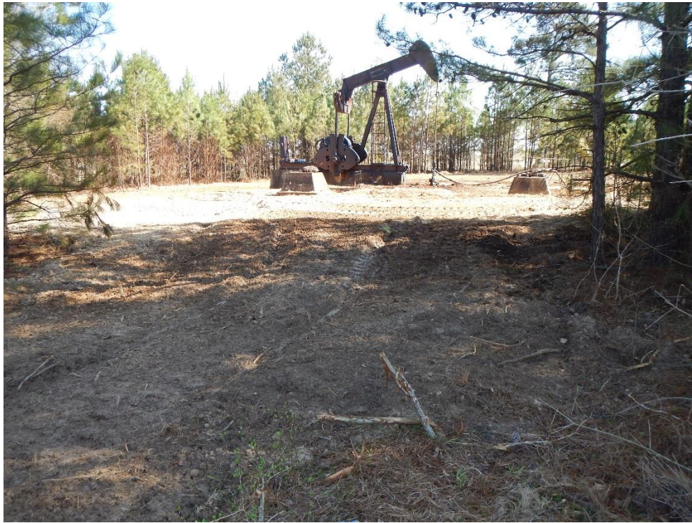
Figure 9. Cleared area for new pump jack installed just outside proposed right-of-way; view is to the south. The cleared area extends into the right-of-way.
