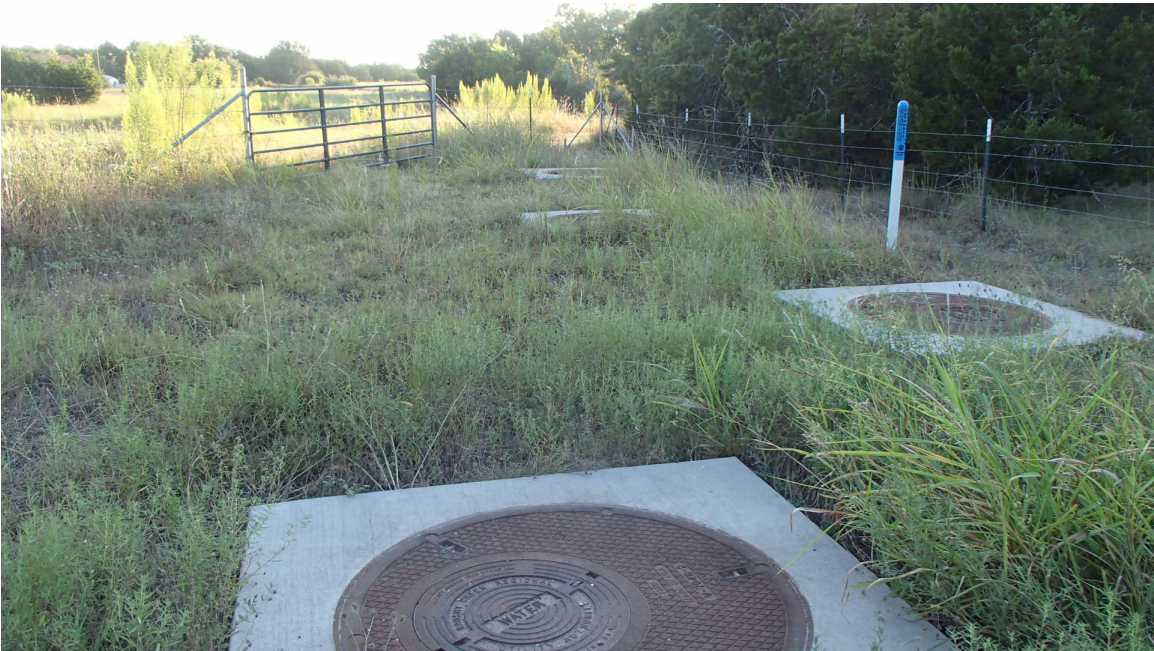
Figure 8. Four of six water mains on west bank of Post Oak Creek, facing east.
