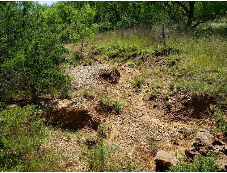
Photograph 49 – Eroded drainage, view to the east.
