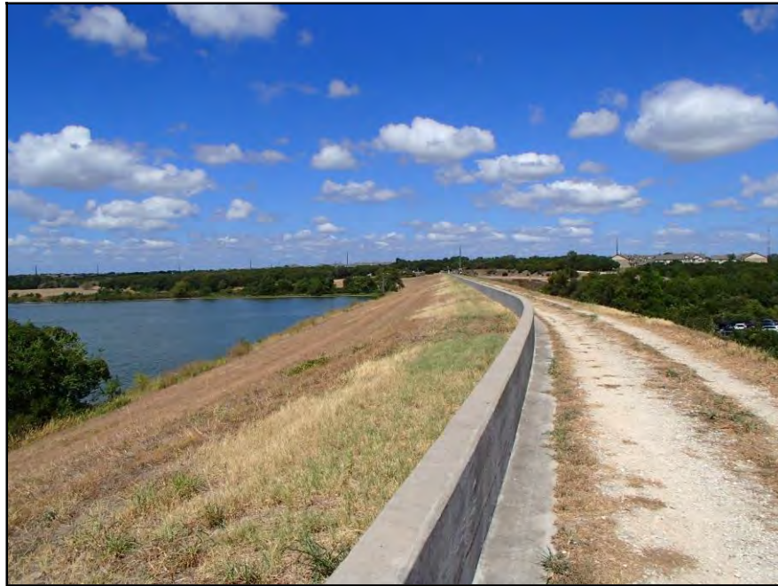
Figure 12. Looking into APE from top of dam in eastern portion of APE; facing northwest
