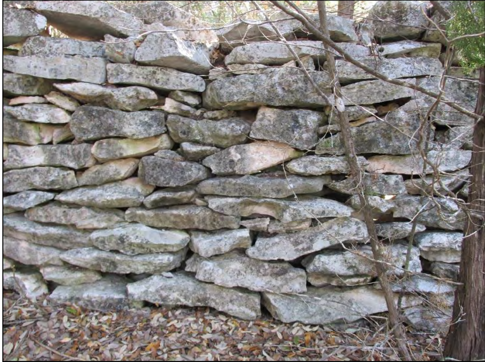
Figure 6. Detail of the north façade of Site 41WM1416 showing an intact portion of the stone wall, coursing to create a stable structure, and chinking.
