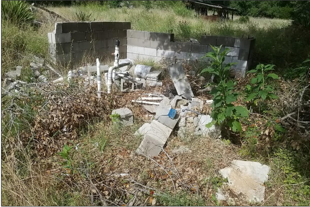
Figure 14. Cinder Block Wall with Modern Water Valve and PVC Piping (Facing Southwest)
