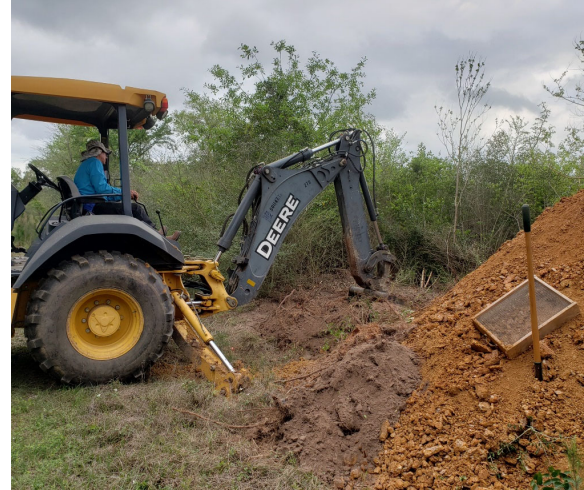
Figure 4-5. Operator Francisco Campusano excavating at T1, using a rubber-tired backhoe with an approximately 1-meter (3-foot) wide-bladed bucket.
