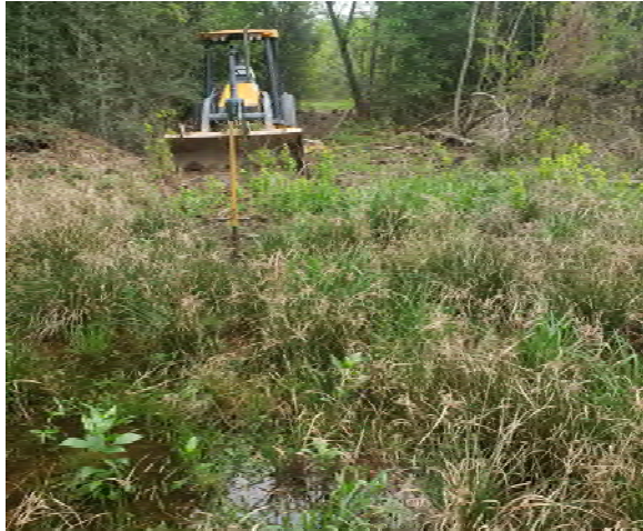
Figure 4-1. Impassable portion of the APE along the inundated path to the planned location for Trench 12.
