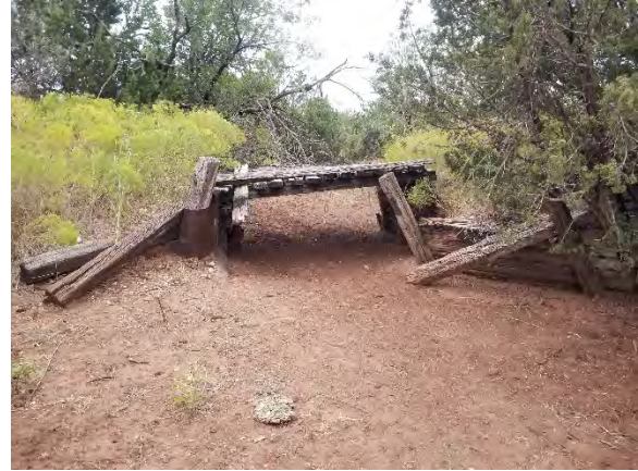
Figure 5-8. Section of berm that crosses the parcel and associated bridge located south of the APE.
