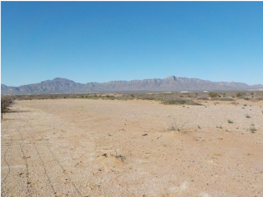
Photograph 4. Overview of area disturbed by waterline construction, facing west, unexcavated shovel test pit noted by orange pin flags.
