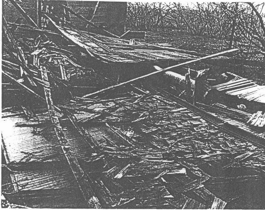
Collapsed roof and wall, west end of house, looking east. Note metal stovepipe and roof ridge.
