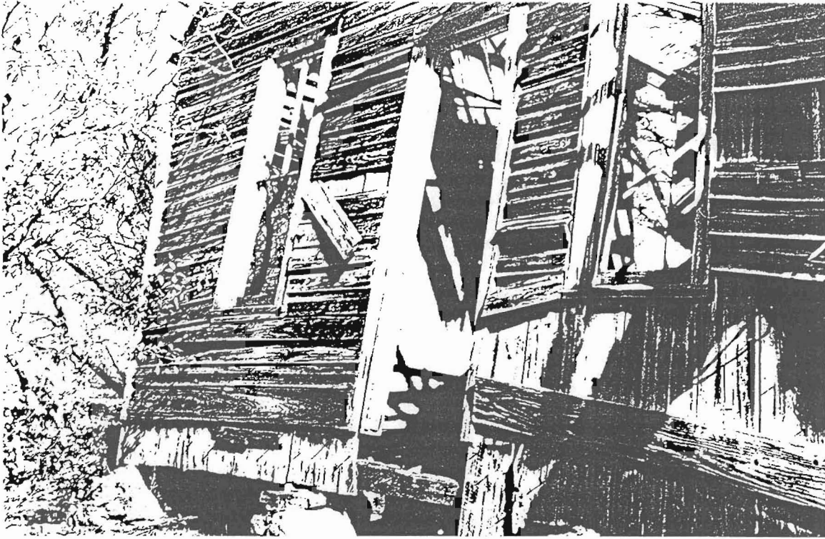
Figure 3A. The house structure was built on sandstone masonry piers and had no stud framework in the walls. The walls are three boards thick; vertical structural boards, carboard interior veneer and exterior horizontal siding.
