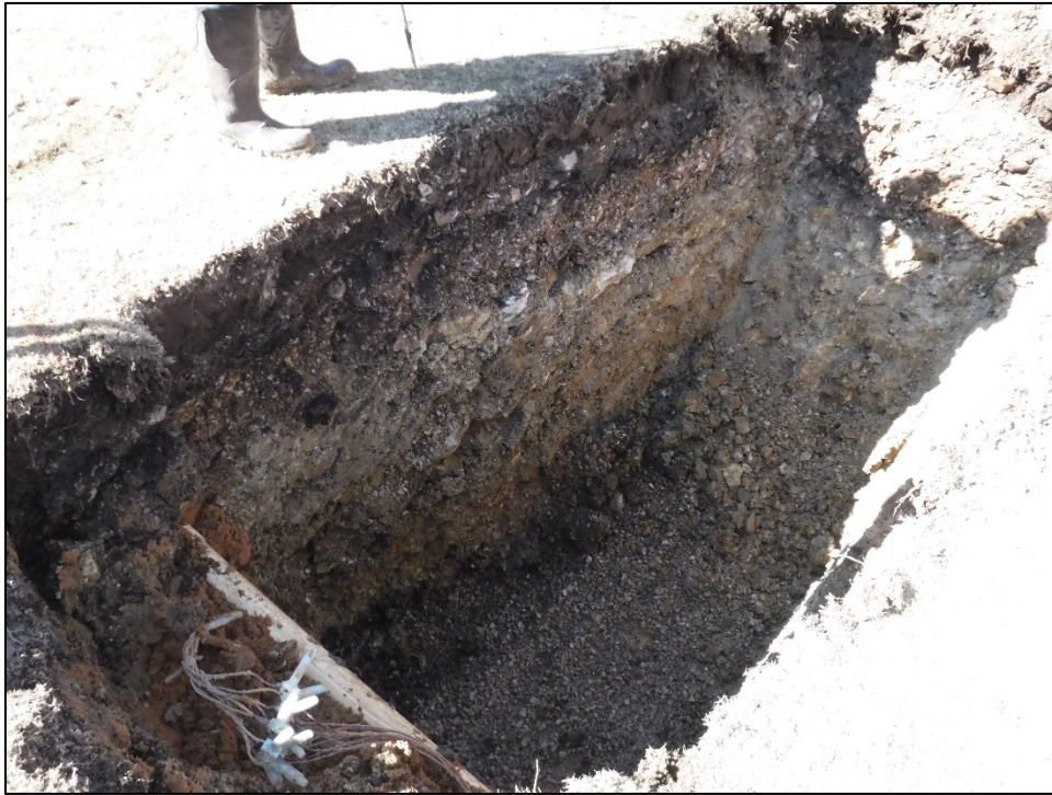
Figure 5-4. Original proportions of BHT1 before collapse, facing northwest.
