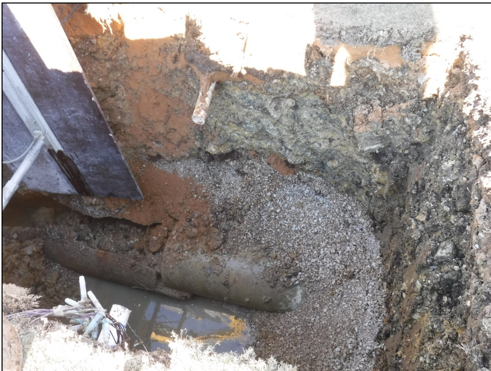
Figure 5-3. Misaligned pipe in BHT1, facing north.
