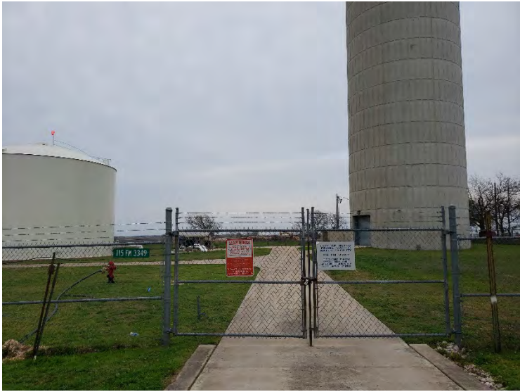
Photograph 19 – Frame Switch PS APE, view to the east.
