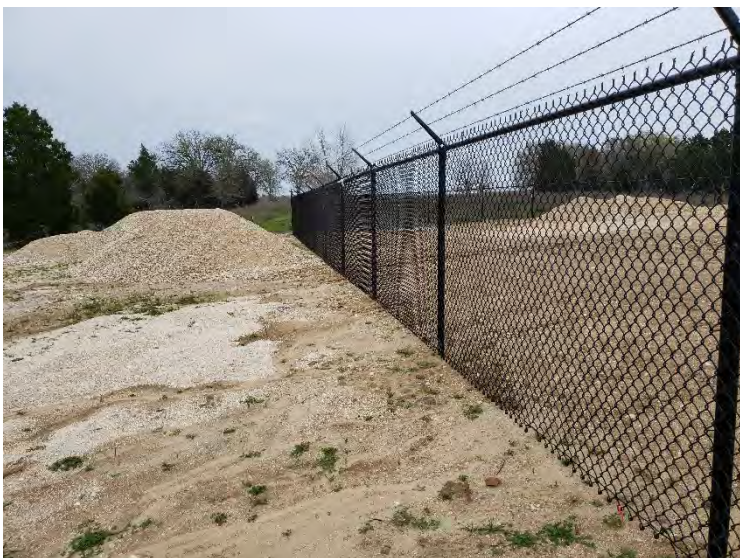
Photograph 23 – Shiloh PS, piles of gravel and dirt within and outside of APE, view to the northeast.
