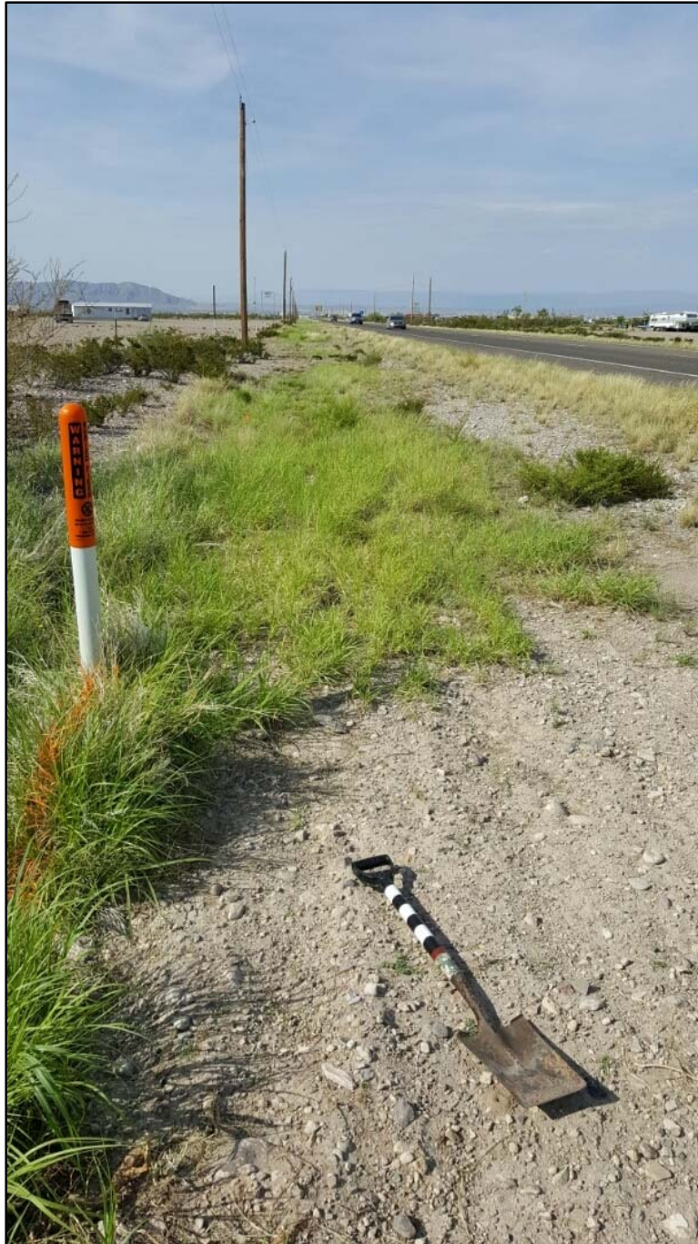
Figure A-6. Buried fiber optic line within the U.S. 67 right-of-way facing southwest.
