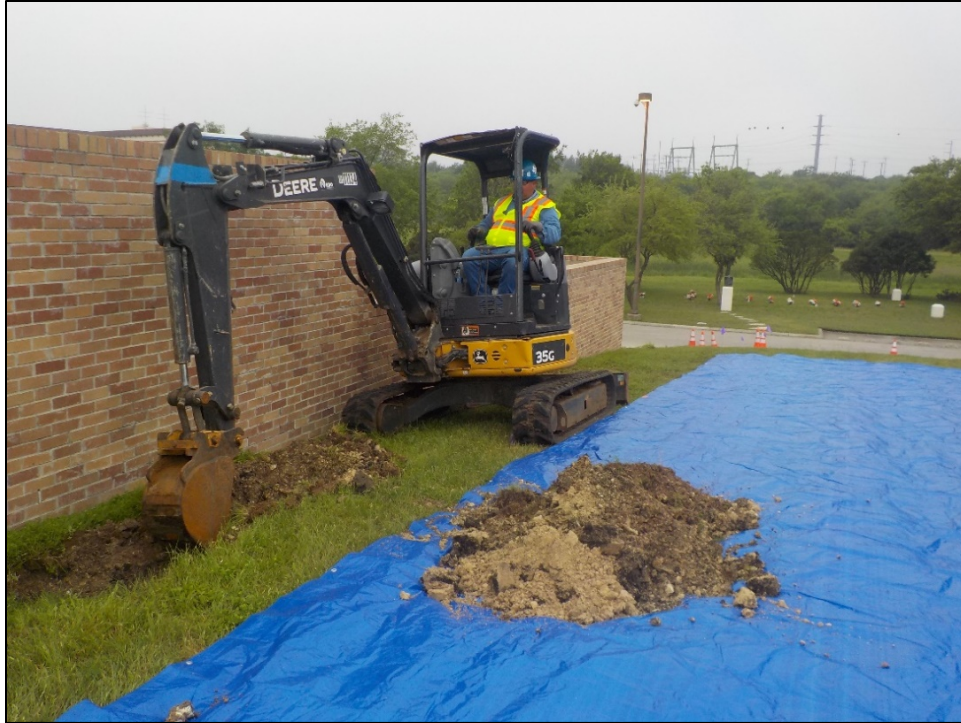
Figure 9. Overview of excavation process within the Project area at Trench 1, view facing west.
