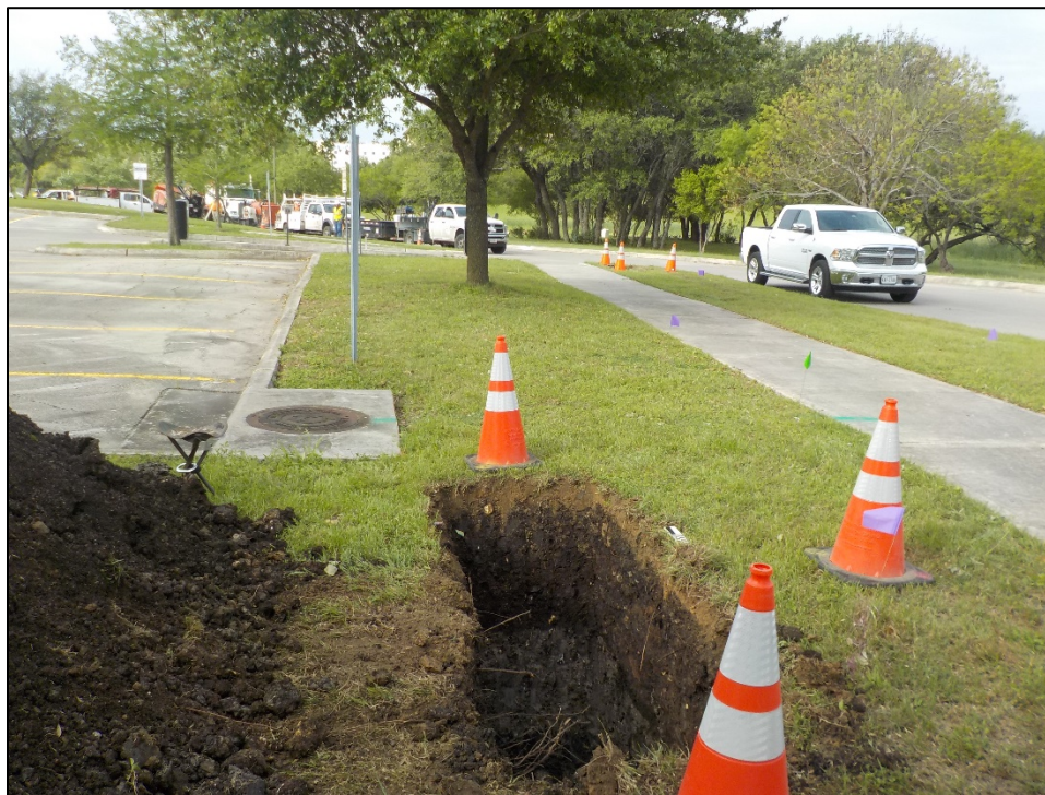
Figure 11. Overview of Trench 7 locale and surrounding disturbances within the Project area, view facing south.
