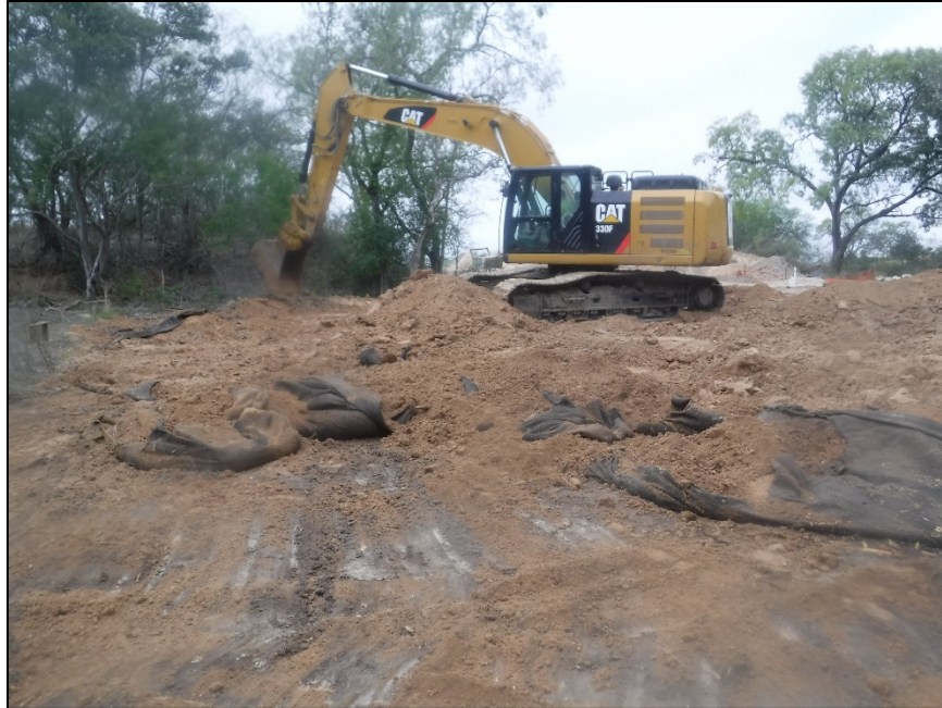
Figure 3. Overview of construction monitoring at site 41GU177 showing the removal of the protective fill layer and geofabric, facing northeast.
