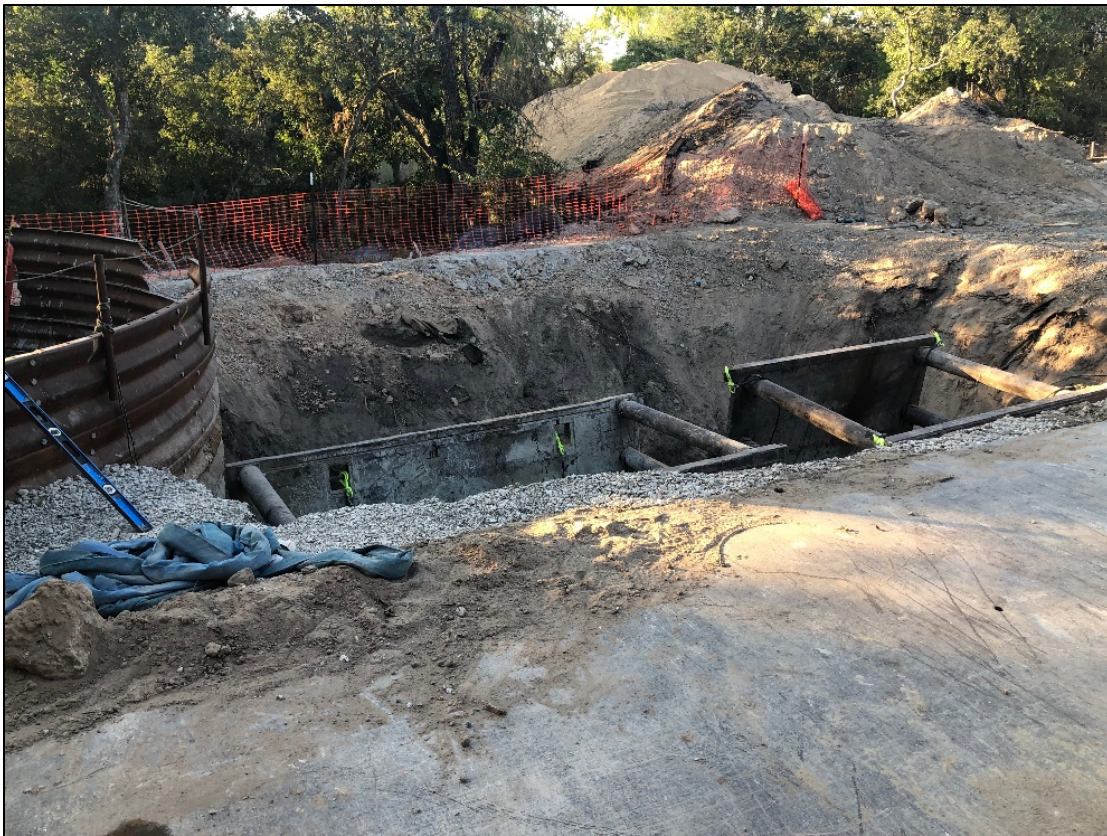
Figure 2. Overview of construction monitoring at site 41GU177 showing shoring placed in trench prior to installation of pipe, facing northeast. Backdirt pile to north was inspected for cultural resources.
