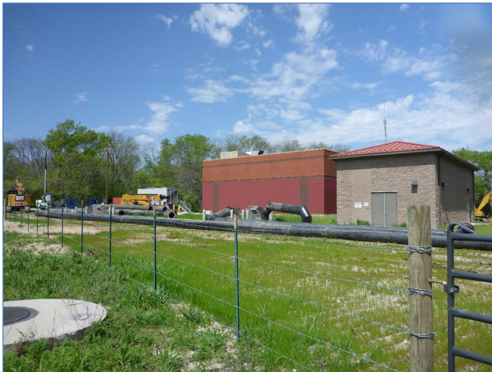
Figure 14. NTMWD maintenance facility construction disturbance in the northeast corner of APE; view northwest.
