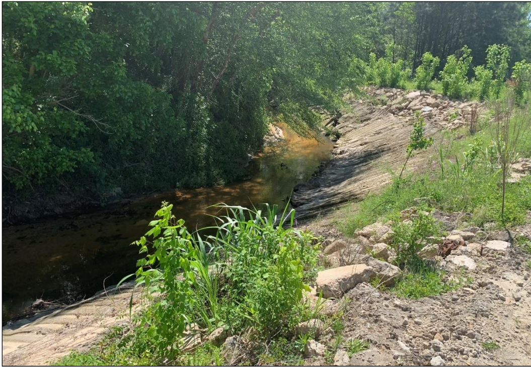
Figure 14. View of Concrete-Lined Banks of Stewarts Creek near Southern End of ROW (Facing Southeast)
