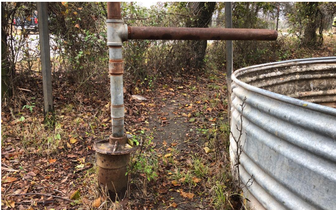
Figure 6-33 Metal piping without output to the stock tank, facing northwest.
