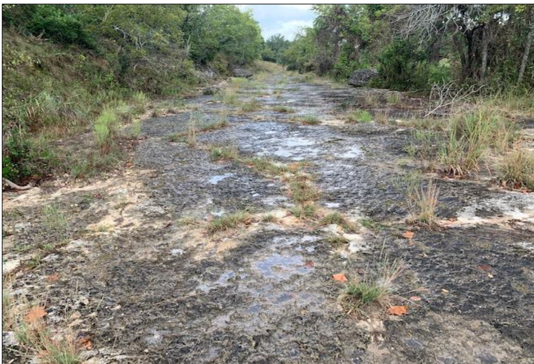
Figure 15. Limestone Step in Central Portion of West Interceptor (Facing North)
