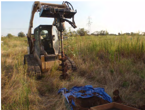
Figure 5-95. Deep testing in progress at Sweetwater Creek, Location DT5. View is to the northeast.
