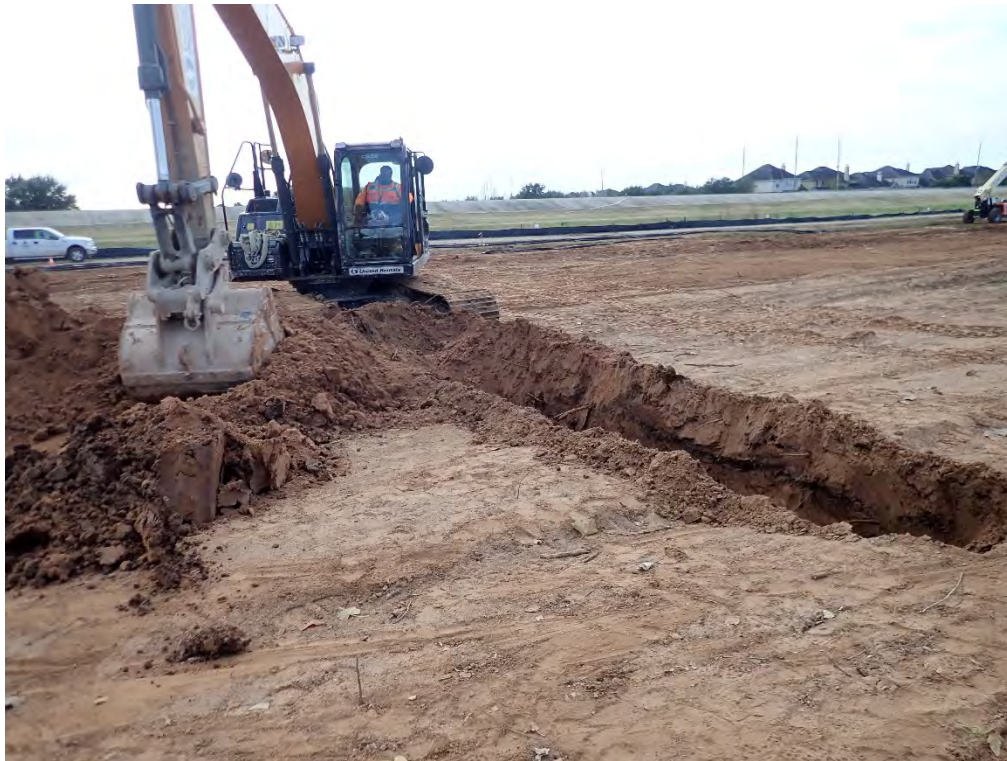
Figure B1. Overview of the Structure 1 location with trackhoe in operation. View is to the south.
