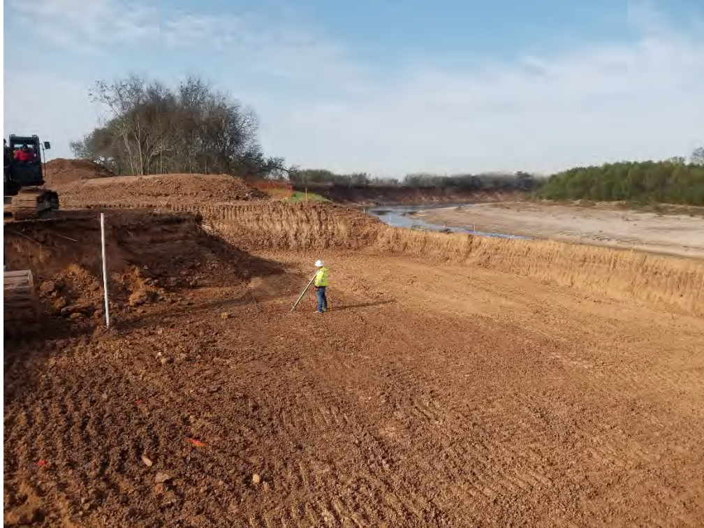
Figure B7. Overview of the excavated Structure 2 location. View is to the west.
