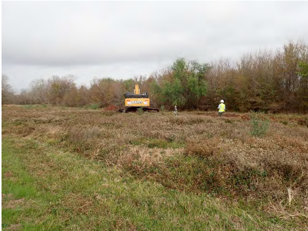
Figure B23. Overview of the Structure 6 location. View is to the northwest.
