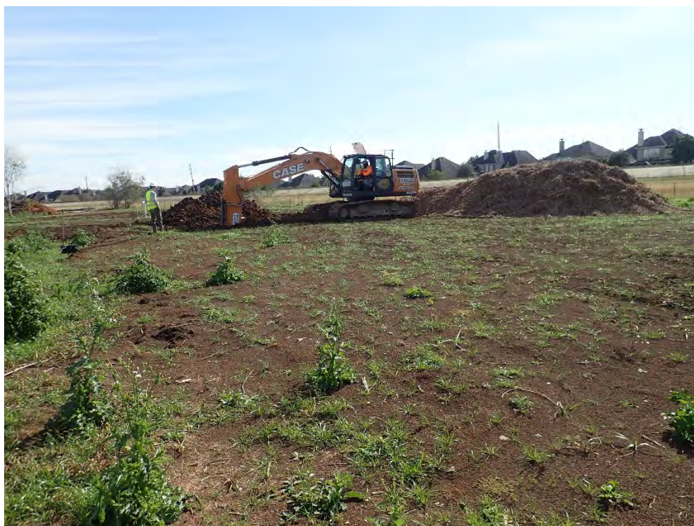
Figure B12. Overview of the Structure 4 location. Note brush pile within the center of the workspace. View is to the southeast.
