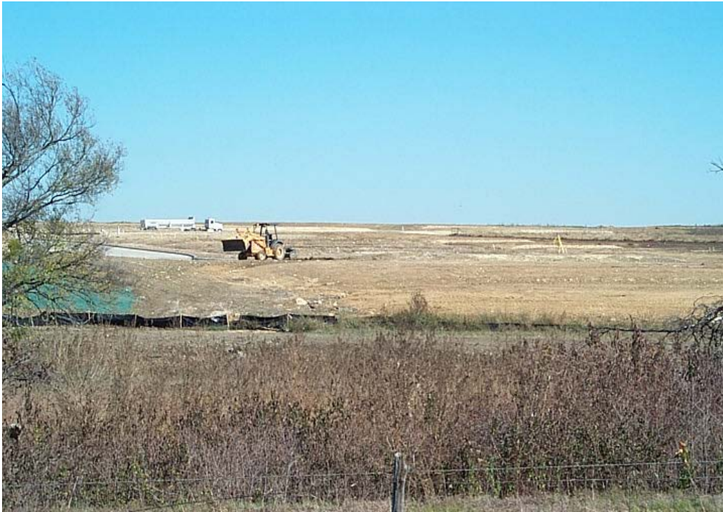
Figure 9. View of construction on the flood plain of Big Fossil Creek east of Blue Mound Road.
