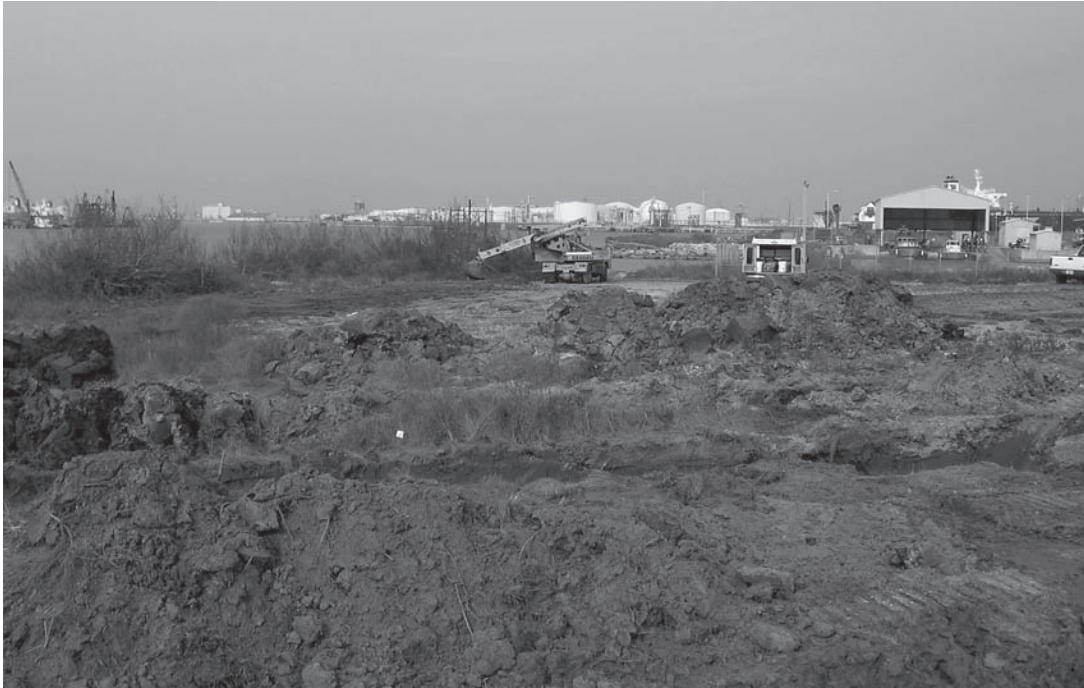
Figure 3.4. View of the southern portion of the project area, looking west. Gradall in background is backfilling Trench 5. Building at right-center is the boathouse at the U.S. Coast Guard Station.
