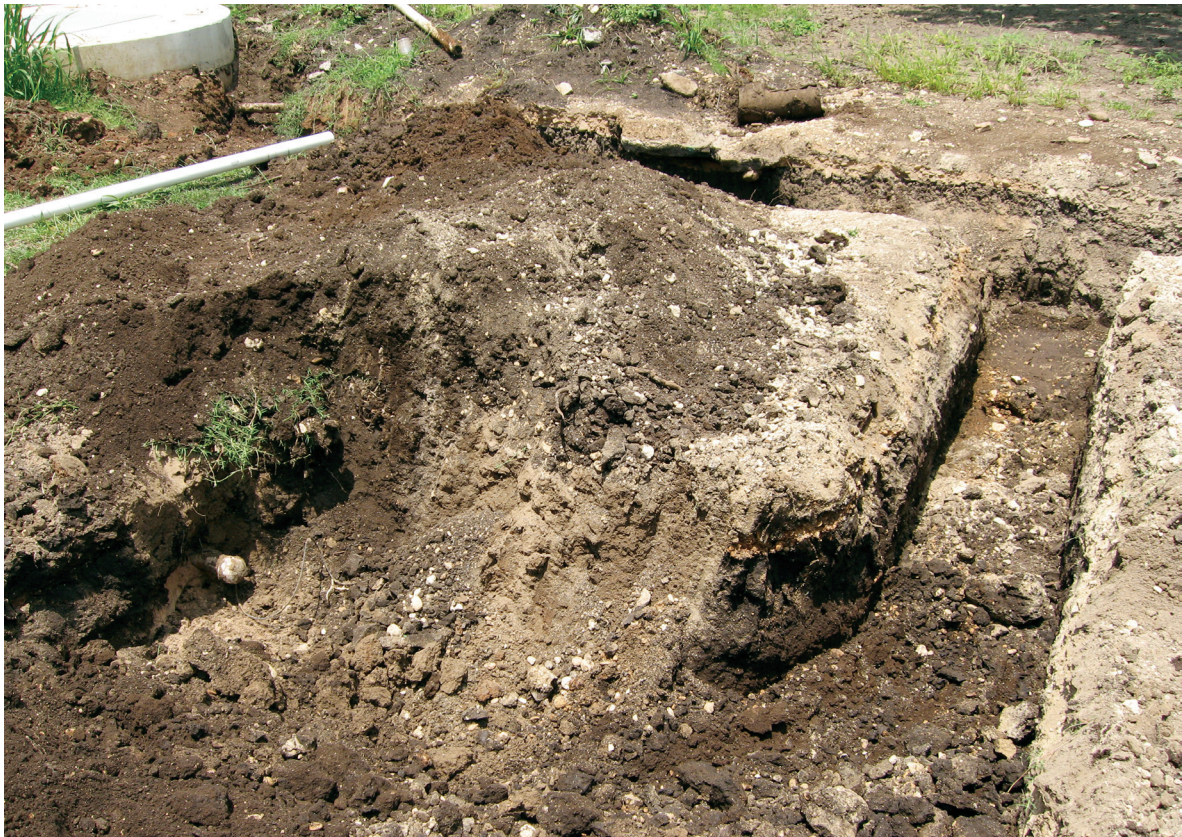
Figure 8-9. Two trenches and one pit for connecting restroom facility with lift station, visible in top left of photo, with new recommissioned irrigation line, facing north.
