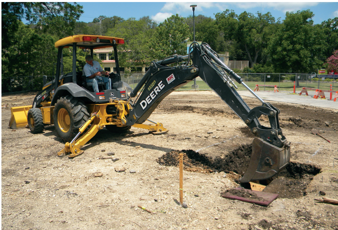
Figure 8-1. Mechanical stripping of an area around Units 3 and 4 in order to trench unit walls for safety. The bottom of excavation units were covered with plywood, visible in photo beneath backhoe bucket, in order to protect unexcavated sediments.
