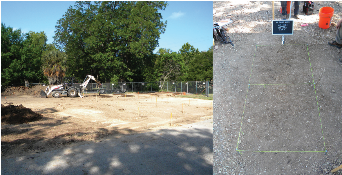
Figure 3-1. Overview of project area after parking surface has been scraped (left) and Units 1 and 2 prior to excavation (right).
