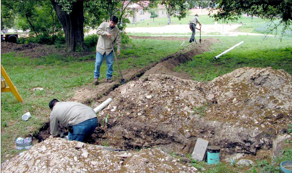
Figure 9-2. Texas State University’s Grounds and Irrigation crewmembers excavating trench adjacent to the President’s House; facing southwest.
