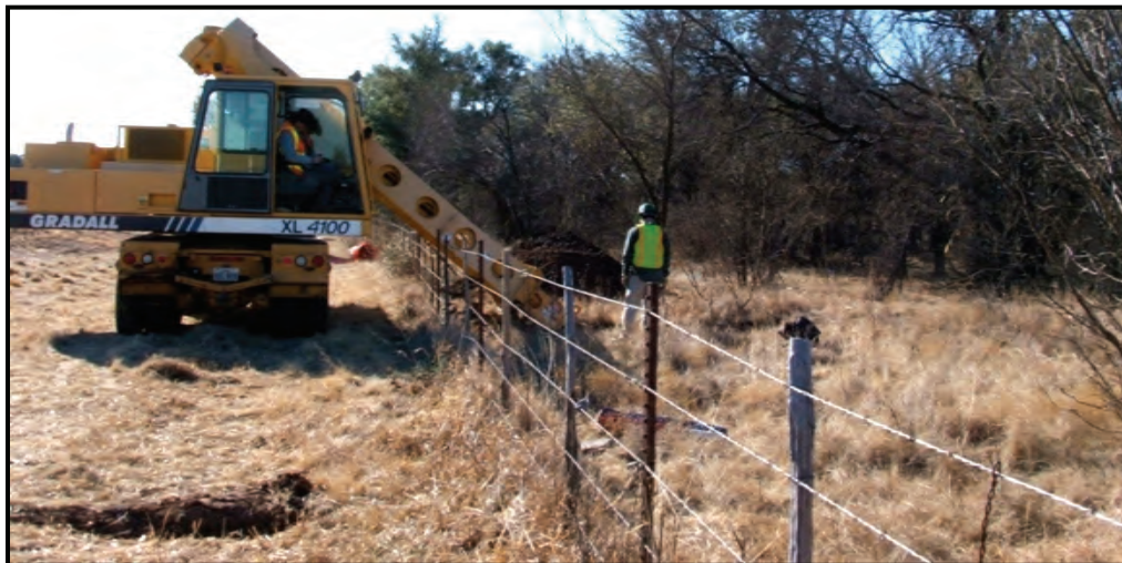
Figure 5-3. View of Gradall® Excavating Trench 4 E/W in proposed New ROW Monitored by TRC Archeologist.
