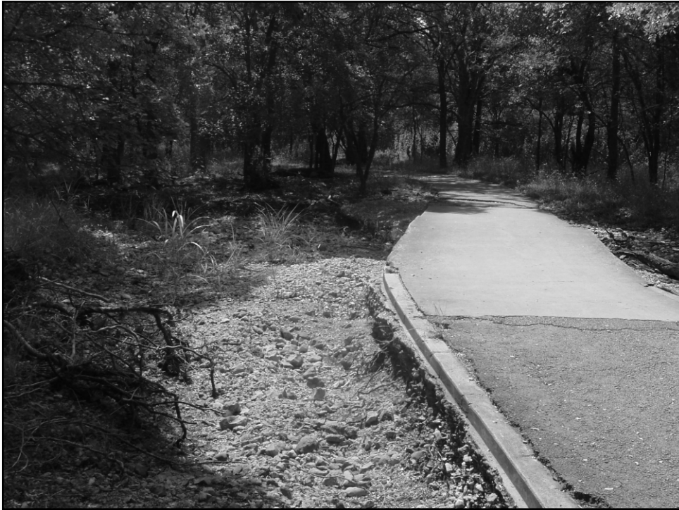
Figure 1-9. Low-water crossing of Lorenz Creek in Area 7. Note erosion at base of sidewalk.
