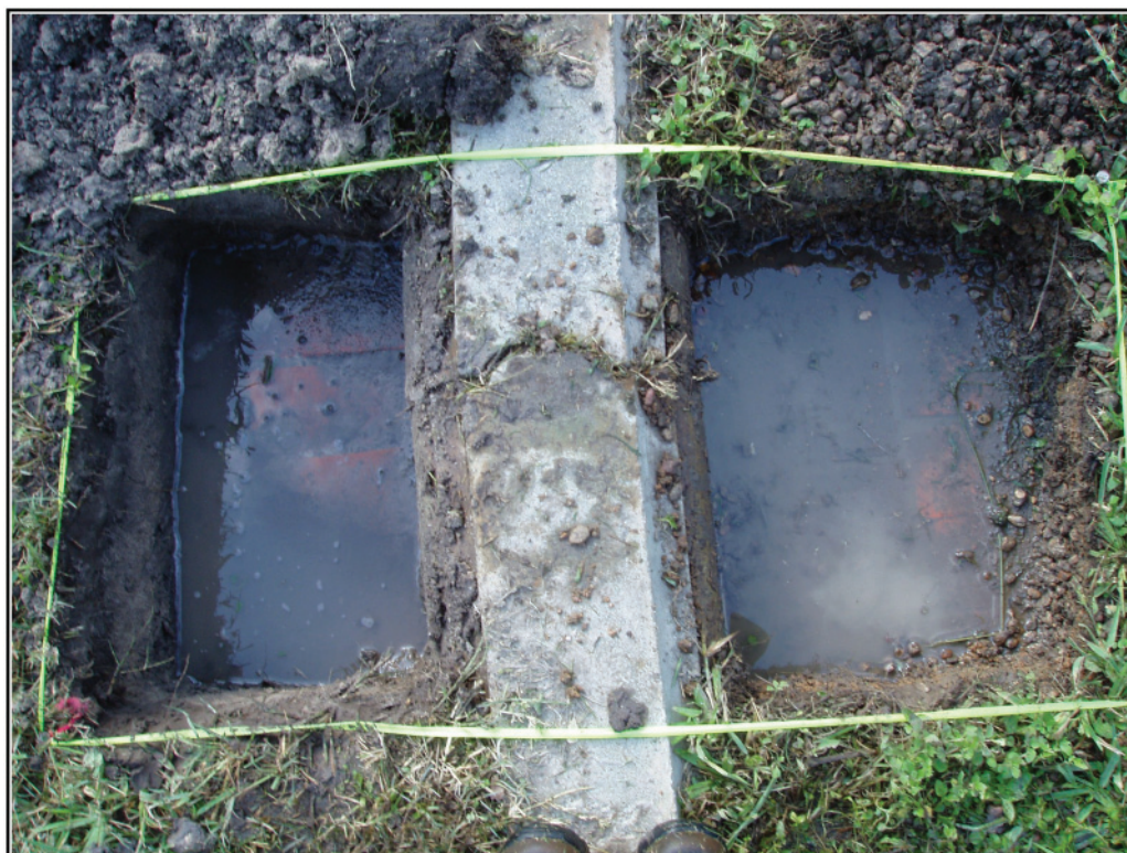
Figure 5-11. Photograph of water seeping into Unit 1 located along the reflecting pool path.
