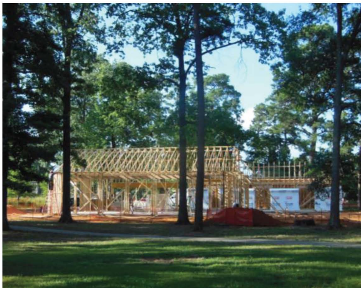
Construction of the new Conservation Education Center is well underway at the Pineywoods Native Plant Center
