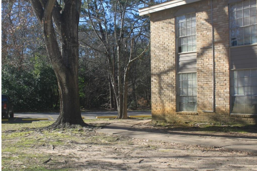
Figure 16: Image showing annual flood level on the side of the University Club Apartments.
