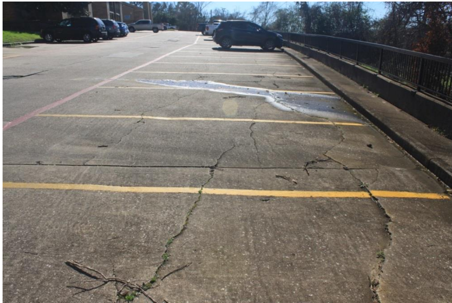
Figure 26: Fractures in the concrete showing the beginning of the development of rotational blocks at the top of the cliff. These fractures indicate that movement is occurring behind the cliff.
