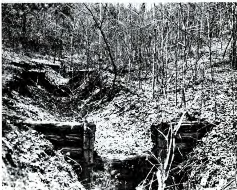
Figure 11. Check dams, as well as vegetation, have an influence in controlling erosion and reducing runoff peak flows.
