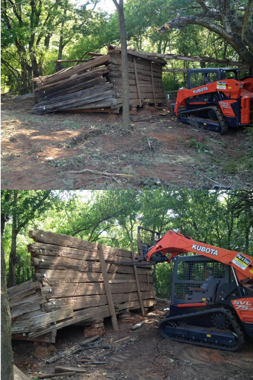
Figure 16: The sides have been removed and boards are numbered (top) and removed (bottom).
