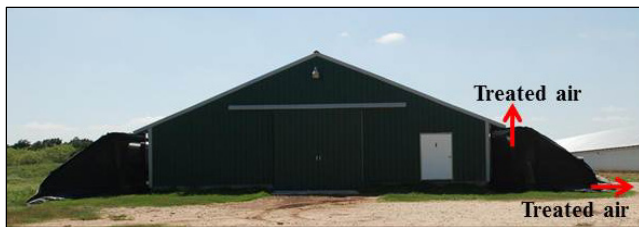
Figure 4. Biocurtain covering the entire exhaust area on both sides of the treatment house. Treated air leaves vertically and through the opening near the bottom corner of the structure.
