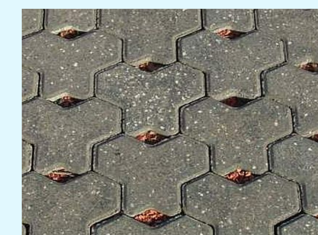
Example of Permeable Pavement
